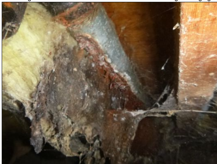
Leak in Drain lines. Under kitchen
