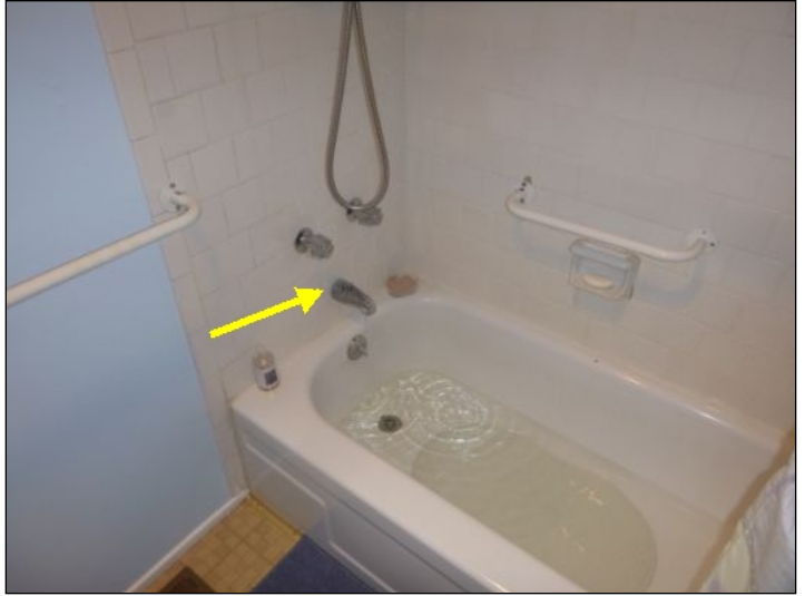
Deteriorating sealant around shower enclosure.
