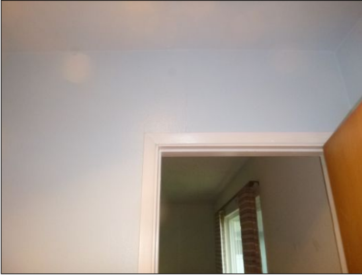
Cracking in wall(s). Master bath
