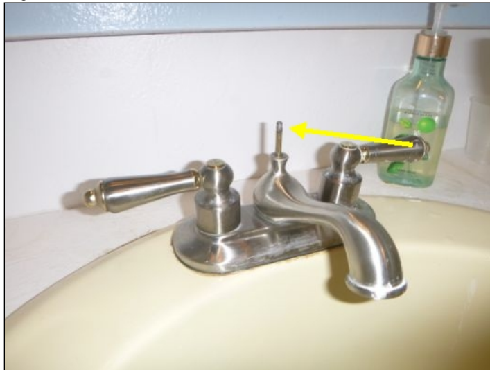
Stopper is missing knob.
