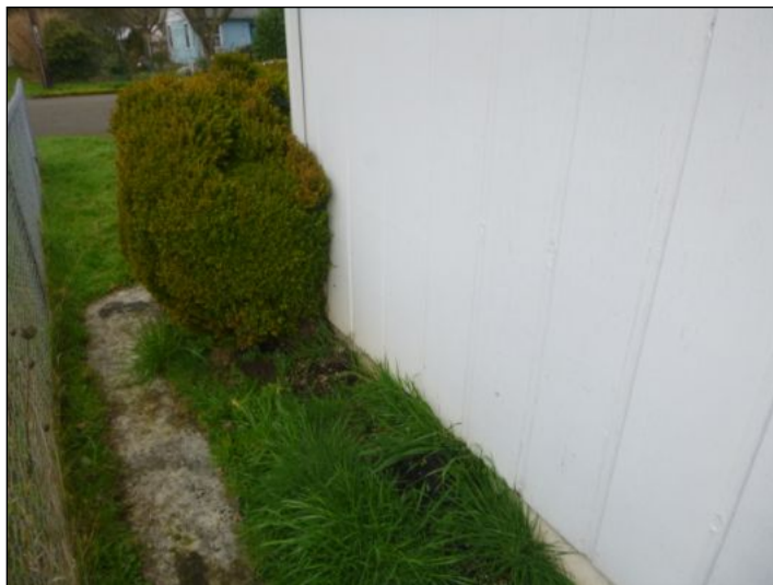
Vegetation within 12" of exterior.
