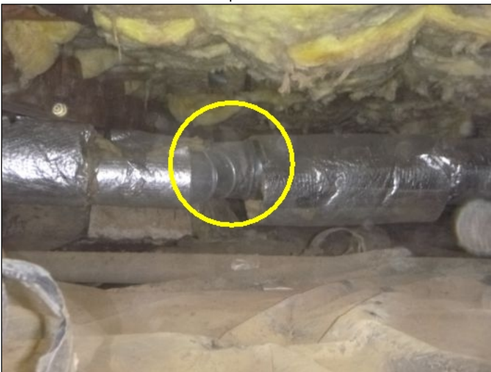
Duct insulation is damaged.
