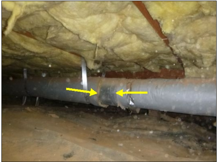
Duct insulation is damaged.
