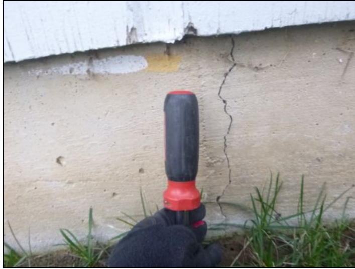
Cracks in foundation.
