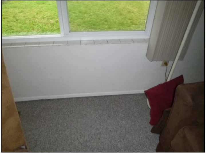
Cracking in wall(s).
