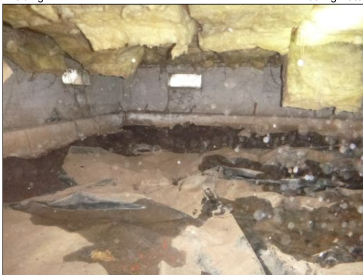
Pooling water in crawlspace. Displaced vapor barrier.
