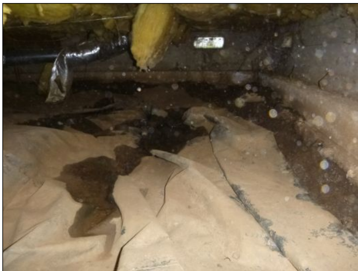
Pooling water in crawlspace.
