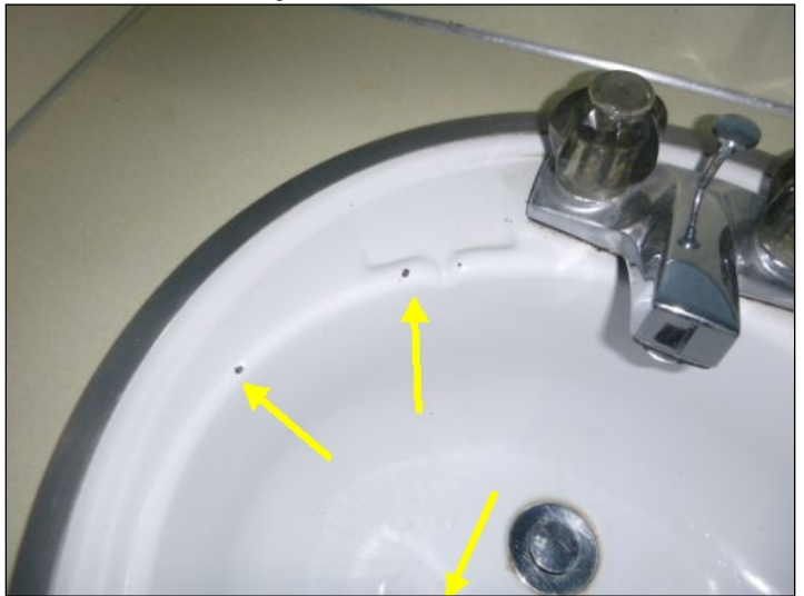
Cosmetic damage to sink.
