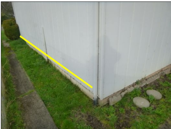
Wood rot in siding
